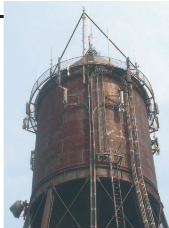
A local water tank doubles as an antenna site for several networks.
